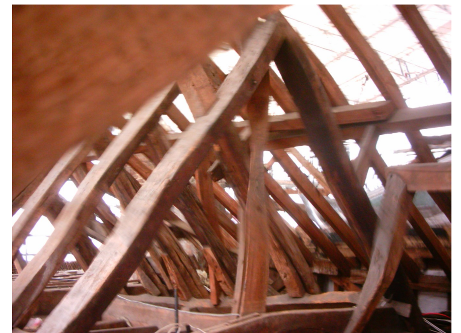
THE BUILDING WAS RE-ROOFED IN 2005: THE PICTURE BELOW SHOWS THE (TRUNCATED) LATE MEDIEVAL ROOF SURVIVING UNDER THE EARLY 19TH CENTURY ONE, IN THE SECTION PARALLEL TO THE PORTSMOUTH ROAD
