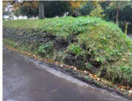
THE CHURCH TRIANGLE—PROBABLY THE TRIGGER FOR THE NEW PROJECT—MAINLY DAMAGE BY LARGE VEHICLES
